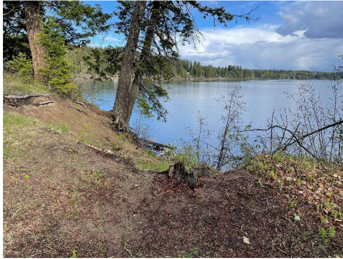
Appendix Photo A-23. Crest of eroding bank on Ness Lake (Restoration Site 1).
