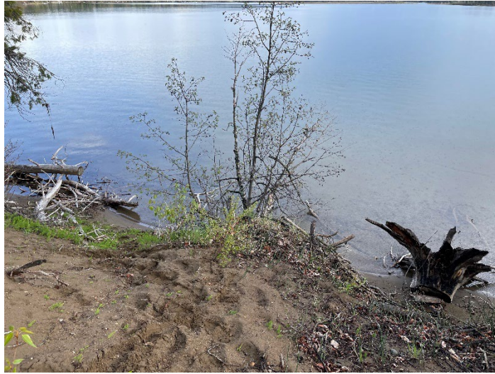
Appendix Photo A-25. Toe of eroding bank on Ness Lake (Restoration Site 1).
