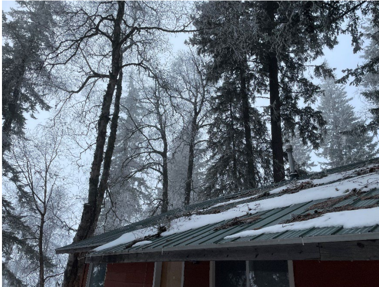
Appendix Photo A-13. Broken limbs from birch trees on cabin roof.
