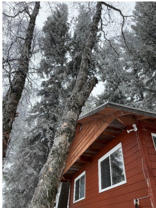
Appendix Photo A-10. Mature birch trees commonly found throughout the camp. Note the cut branch that once leaned over the cabin. It is likely that this entire tree will need to be cutdown in the future since it is leaning toward the cabin.
