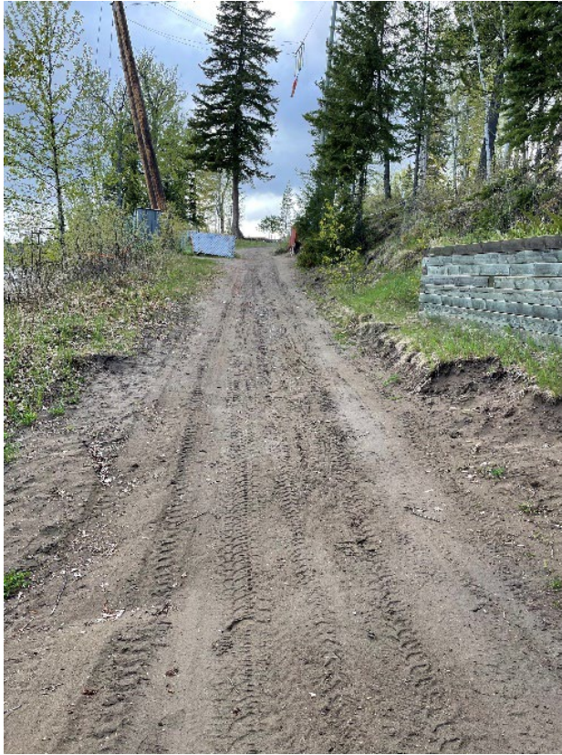
Appendix Photo A-21. Uphill view of road that leads to the beach. Note the sand surface that needs monitoring and maintenance, so sediment does not get transported to Ness Lake from this section of road. Three shallow water bars or berms will be installed to direct water to the roadside vegetation.
