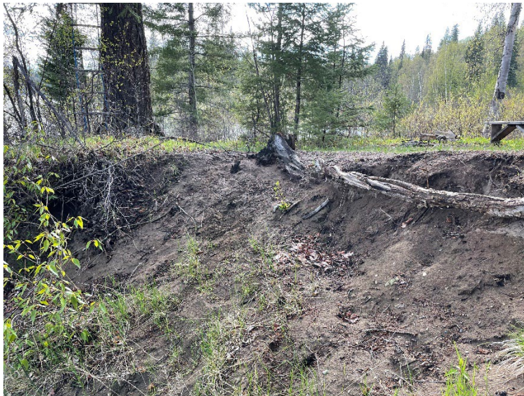
Appendix Photo A-22. Crest of an eroding bank on Ness Lake at Campsite 9. Note: This campsite has been closed to campers and will be restored (Restoration Site 1).
