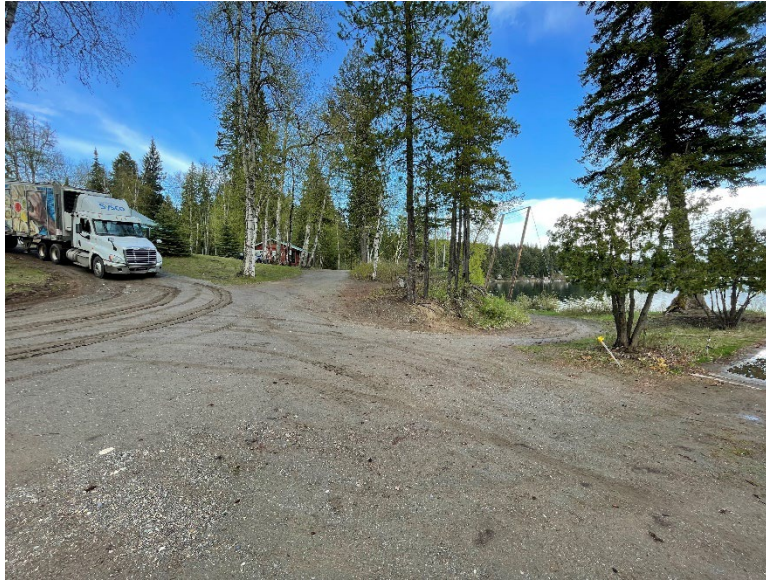
Appendix Photo A-17. Road maintenance is required to make sure the road surface is suitable for traffic and that sediment transported from the road network can't enter environmentally sensitive areas.
